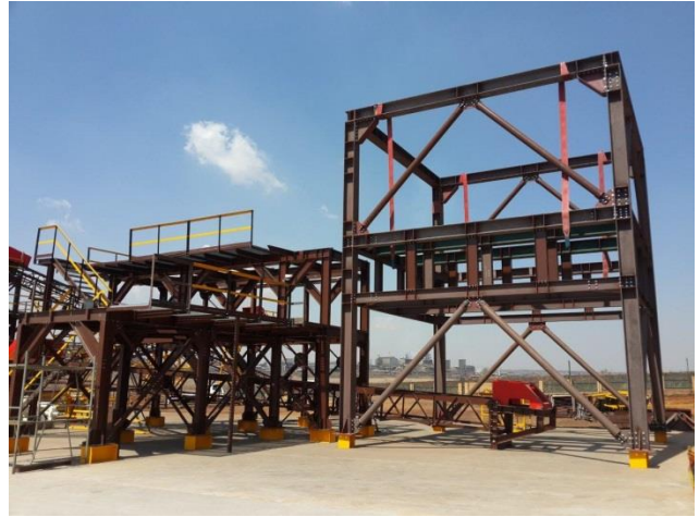
BC1/BC2 primary crushing and screening module structure prior to inclusion of sub-assemblies
