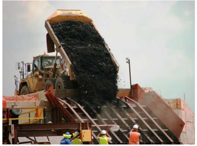
First coal tipping into the plant
