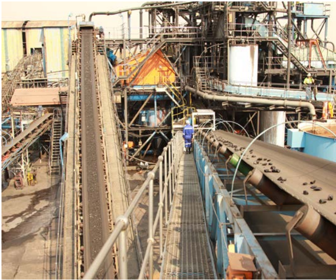
Above: The first NCC Coal Handling and Processing Plant being re-commissioned with the arrival of ROM coal from the underground operation
